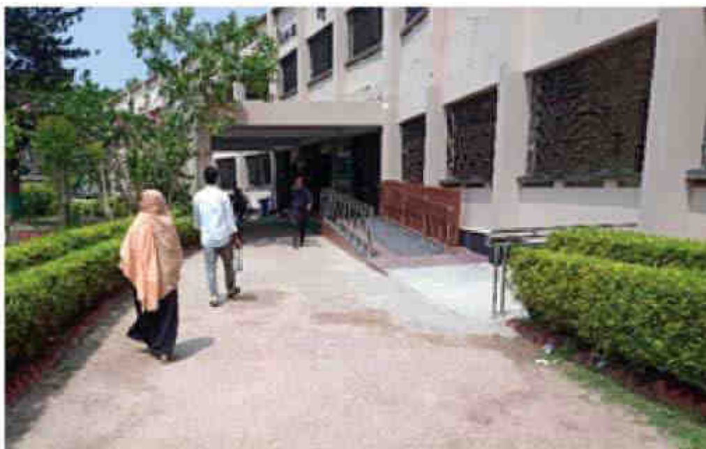
An accessible front entrance of an eye-hospital in Narshingdi after the installation of a ramp.
