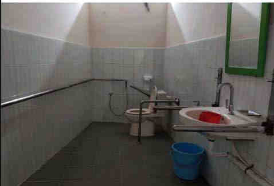
An inside view of an accessible toilet of an eye-hospital with necessary modification and installation in place.
